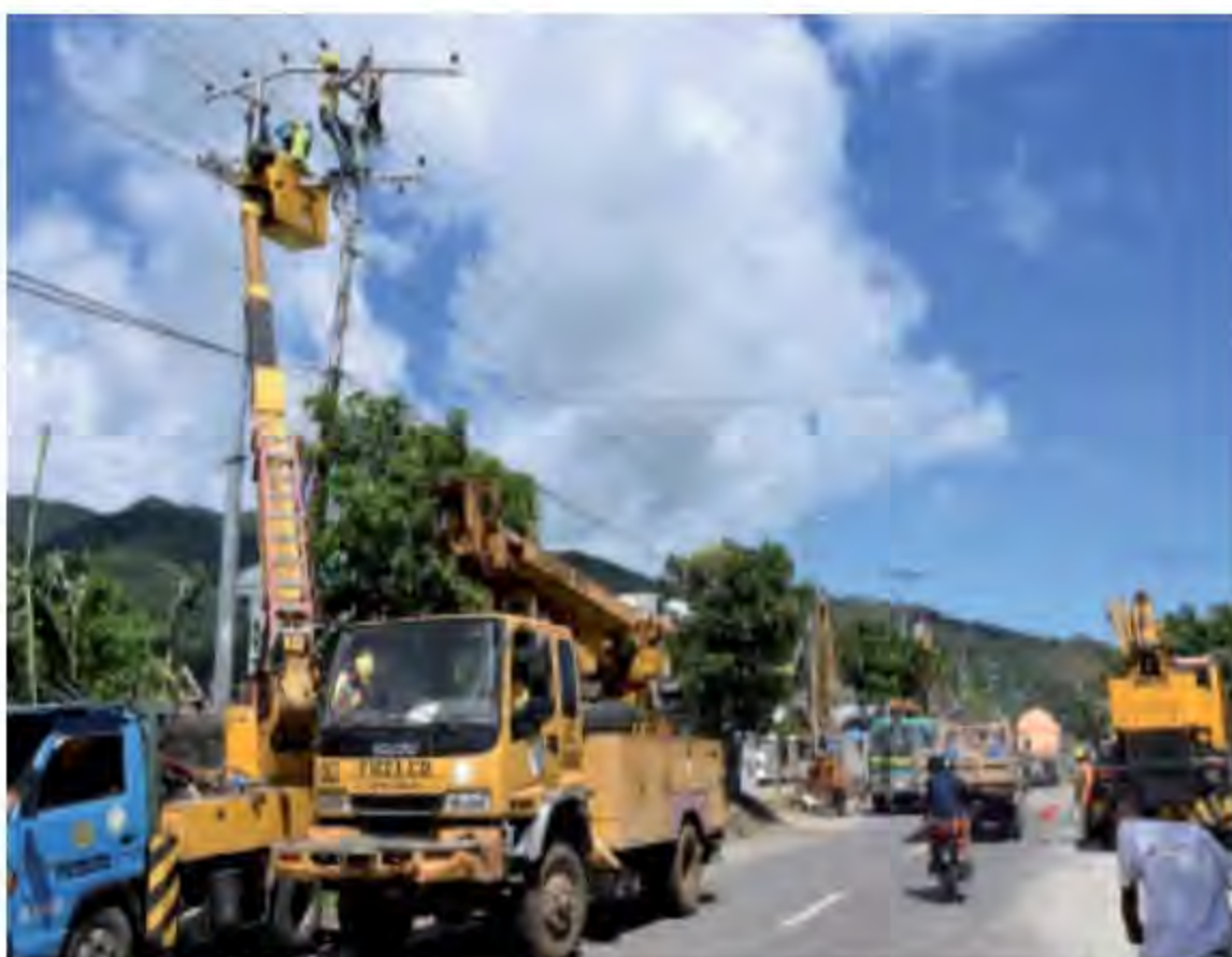
Line rehabilitation and power restoration works being done in the Province of Catanduanes
